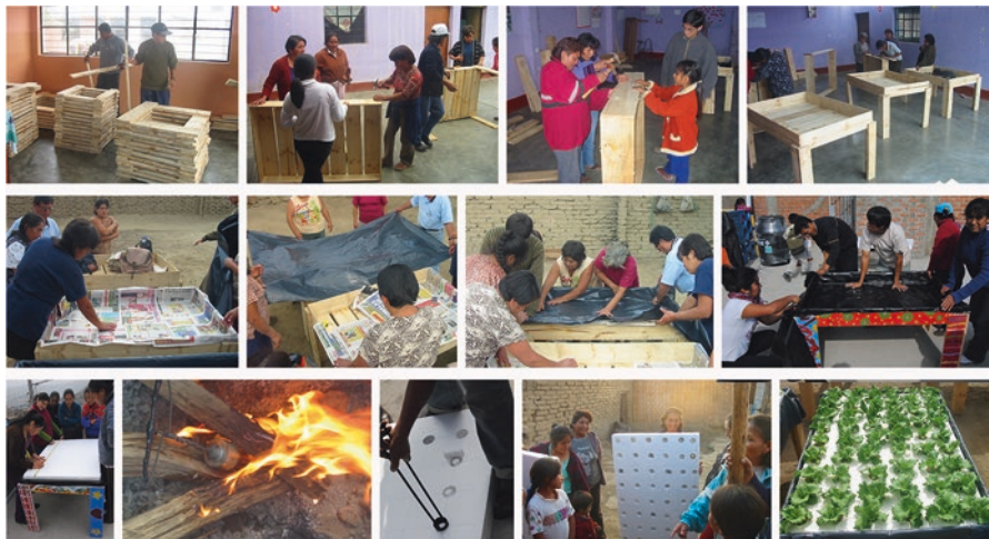
Fig. 5 Step-by-step procedure for building up a simplified floating system. Top row , construction of the growing table. Middle row , insulation and waterproofing with a black PE film. Bottom row , preparation of the styrofoam trays by making holes with a hot iron rod. Images from Lima and Trujillo, Peru (Photo: F. Orsini)
