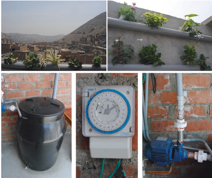
Fig. 2 Modified NFT system that works with a pump in the children playhouse at Monterrey, Lima, Peru (Photo: F. Orsini). Top , views of the hydroponic gardens, bottom, left to right , tank for the nutrient solution, electric timer and hydraulic pump
